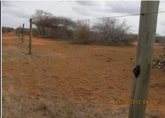
A broken part of the fenceline along Murondo Dakota stretch.
